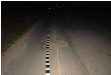
FIG. 6 The cavity which caused the loss of steering stability)
