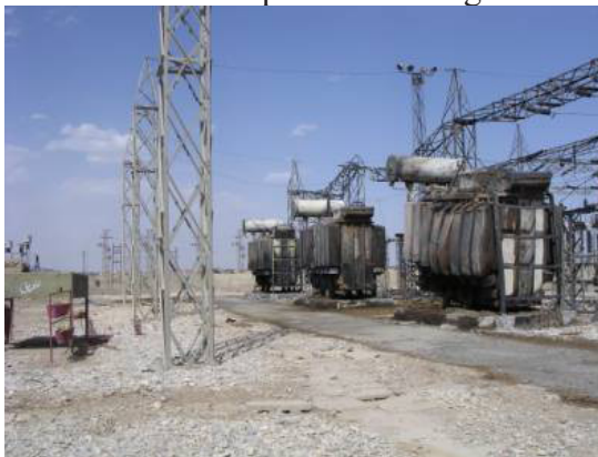
Fig.1 The 400 kV Electrical Power Transformer Station bombed by U.S. Air Force in Nasiriyya on March 22, 2003, with a carbon fiber bomb (Source: R. E. Brigety, Human Rights Watch, 2003, [4])
